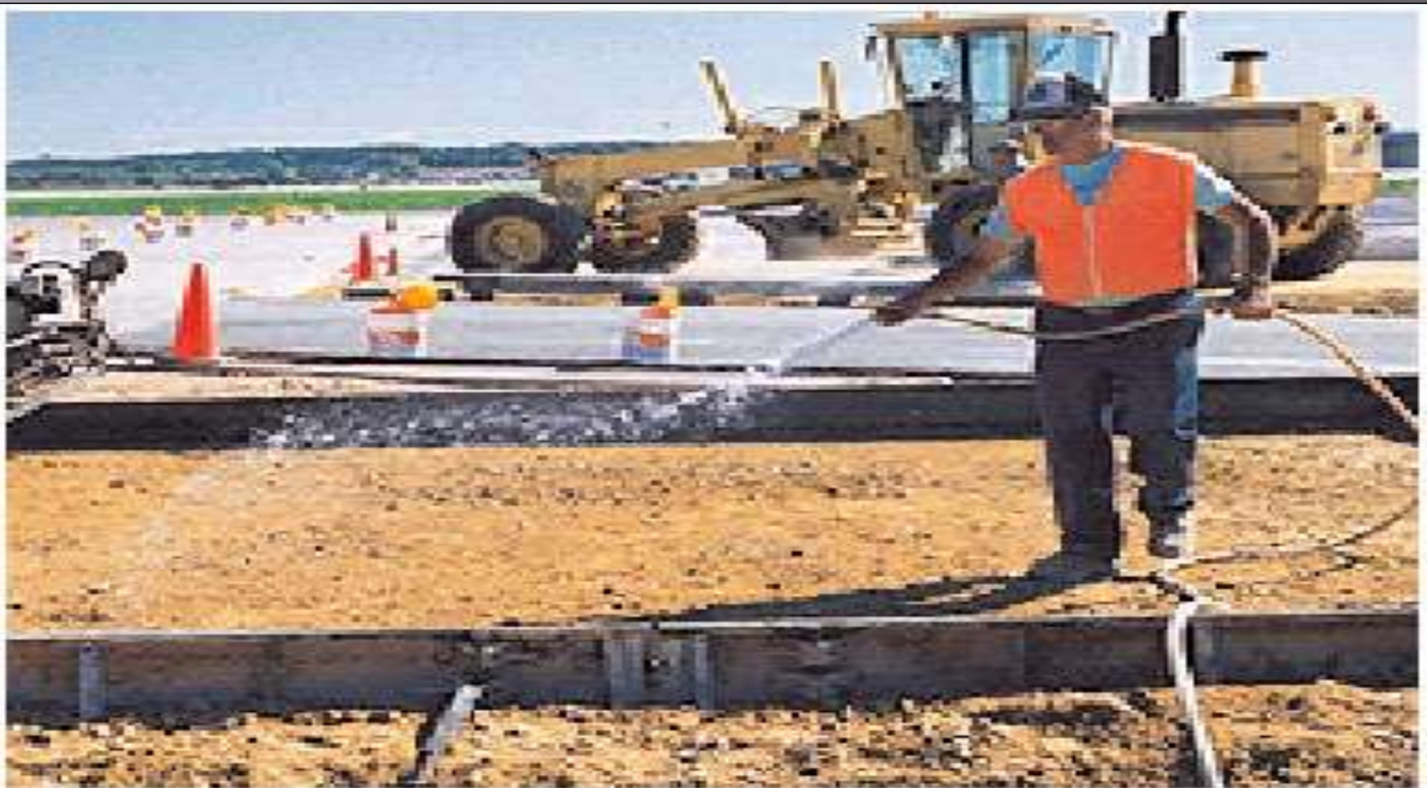
Fig. 13-9. Dampening the subgrade, yet keeping it free of standing water will lessen drying of the concrete and reduce problems from hot weather conditions. (69955)
